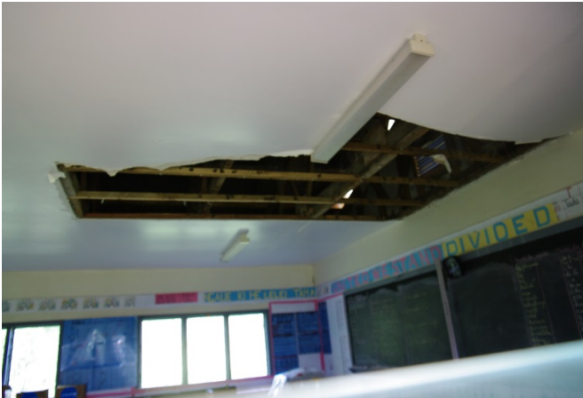
Figure 37 Lost Ceiling in main classroom block at Fotua Government Primary School
