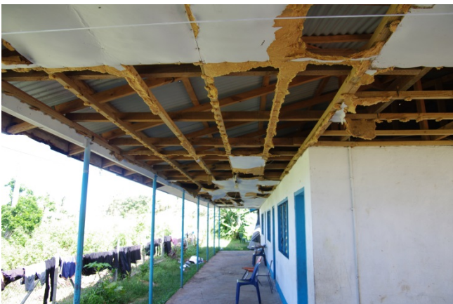
Figure 81 Damaged Ceiling in the Secondary Classroom Block at Ofamo’oni Primary and Secondary School
