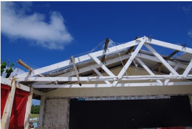
Figure 69 Destroyed Classroom Building at Mo'unga'one Government Primary School
