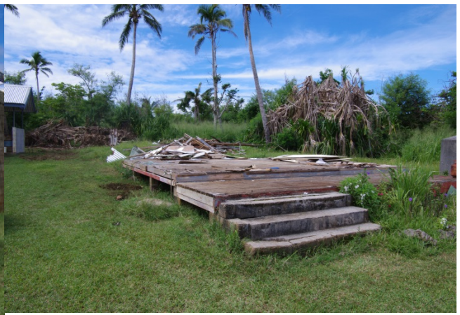
Figure 40 Small Classroom that was destroyed at Fotua Government Primary School
