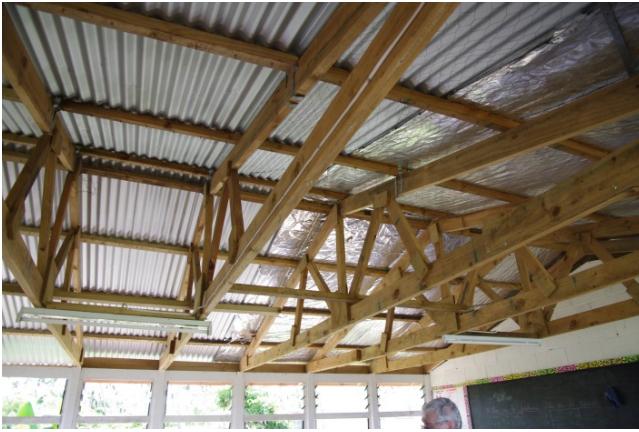
Figure 31 Missing Ceiling in the Classrooms of Faleloa Government Primary School
