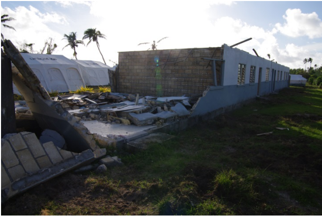
Figure 43 Collapsed wall in the classroom block at Fakakai Government Primary School
