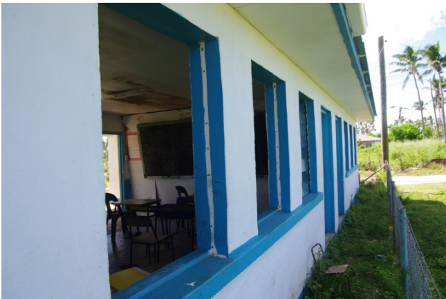
Figure 79 Damaged windows in the Primary Classroom Block at Ofamo’oni Primary and Secondary School
