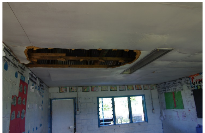
Figure 82 Damaged Internal Ceiling in the Secondary Classroom Block at Ofamo’oni Primary and Secondary School
