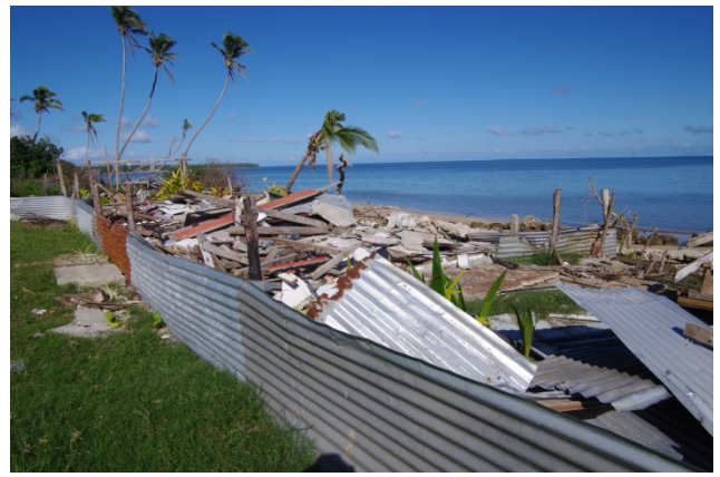
Figure 100 Cyclone Debris placed within the coastal zone at Tailulu College Free Church of Tonga School
