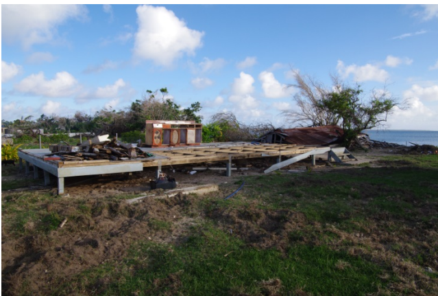
Figure 45 Destroyed Residential Building at Fakakai Government Primary School
