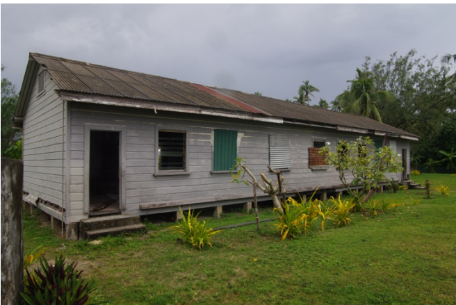
Figure 63 Proposed Kindergarten with Asbestos Roof at Mata'aho Government Primary School
