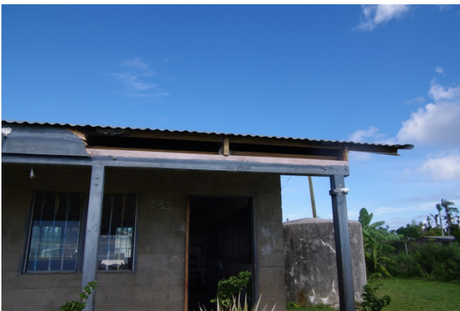
Figure 27 Tongoleleka Government Primary School – Lost fascia and guttering
