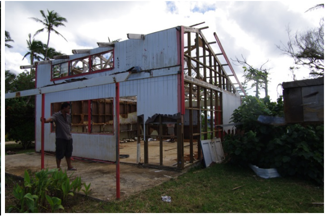
Figure 18 Koulo Government Primary School - building destroyed by Tropical Cyclone Ian
