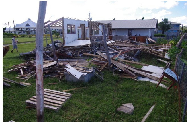
Figure 98 Destroyed Third Classroom Block at Tailulu College Free Church of Tonga School
