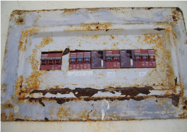
Figure 75 Rusted Electrical Switch Board at Ha'apai High School Hall
