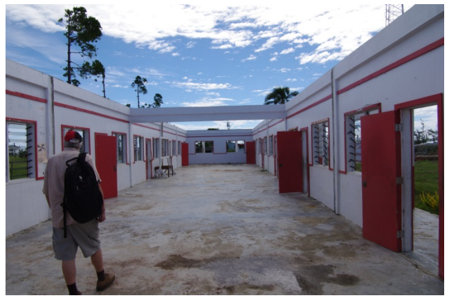
Figure 22 Pangai Government Primary School – Second Classroom Block that has been totally destroyed
