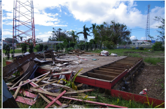
Figure 24 Destroyed Small Classroom at Pangai Government Primary School
