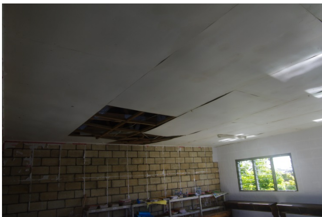
Figure 49 Internal Damage to main classroom building at Ha'ano Government Primary School
