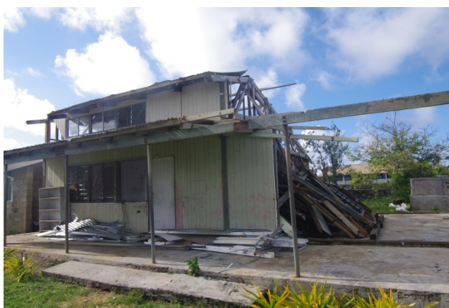
Figure 52 Destroyed Building at Ha'ano Government Primary School
