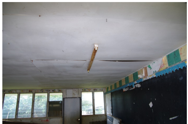
Figure 16 Internal Ceiling Damage to older Japanese Designed Classroom at Koulo Government Primary School
