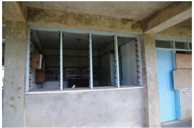
Figure 92 Missing Louvers in Main Classroom Block at St Joseph's Roman Catholic Church School
