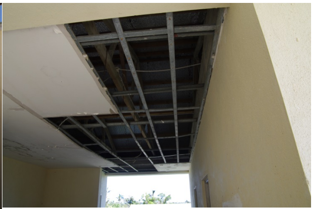
Figure 74 Damage Ceiling at Ha'apai High School
