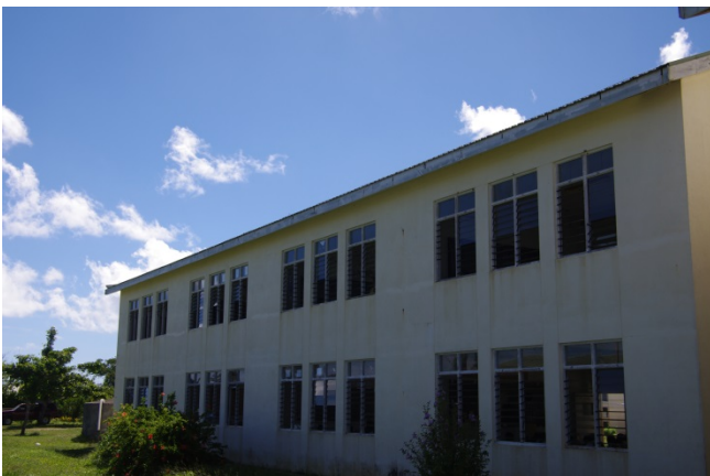
Figure 73 Lost Gutters on Classroom Building at Ha'apai High School Hall
