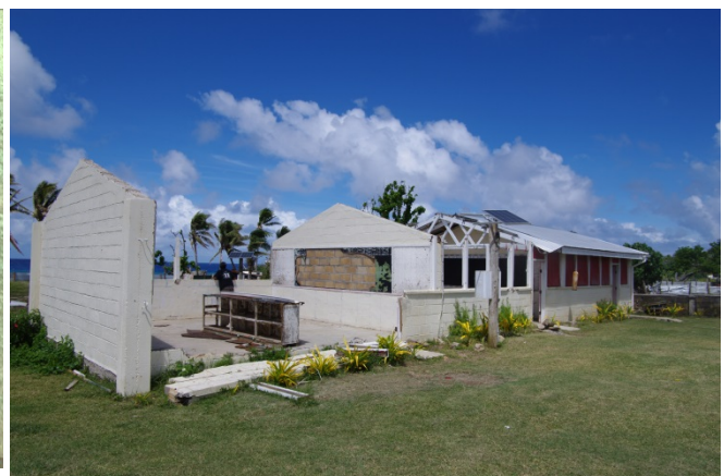
Figure 66 Destroyed Classroom Building at Mo'unga'one Government Primary School
