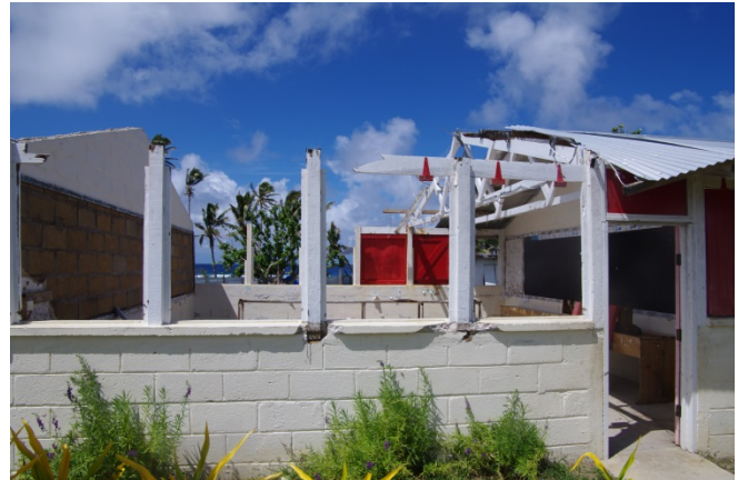
Figure 68 Destroyed Classroom Building at Mo'unga'one Government Primary School
