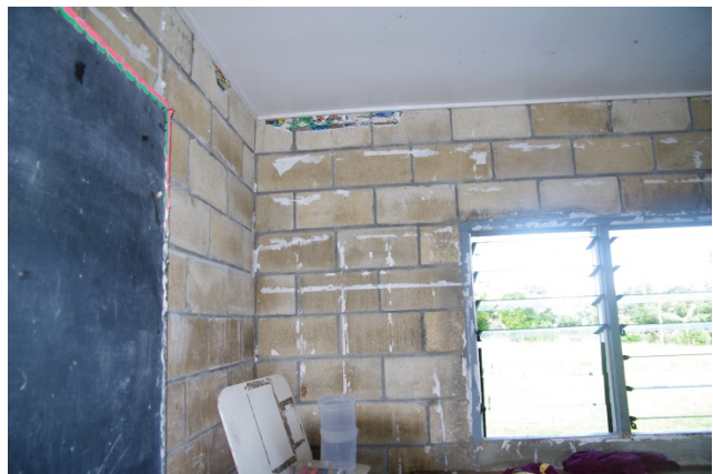
Figure 28 Water damage in northern classroom at Tongoleleka Government Primary School
