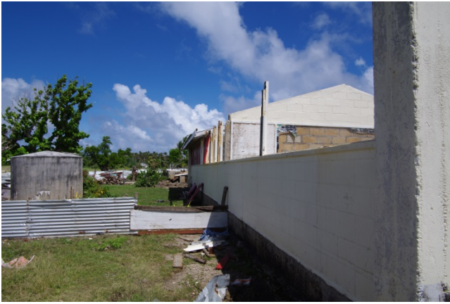
Figure 67 Destroyed Classroom Building at Mo'unga'one Government Primary School
