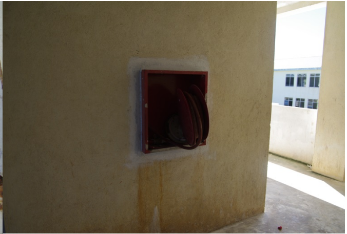
Figure 76 Damaged Fire Hose at Ha'apai High School
