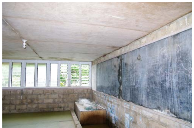
Figure 58 Water Damage to a classroom at Lofanga Government Primary School
