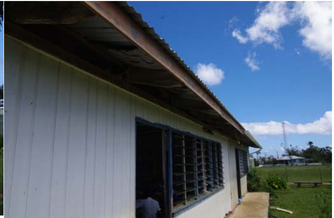
Figure 86 Missing Gutter on Main Classroom at Petani Bilingual Free Wesley Church School
