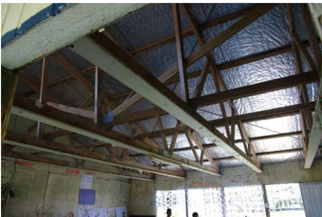
Figure 87 Damaged Ceiling in Main Classroom Building at Petani Bilingual Free Wesley Church School
