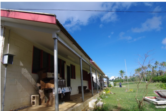
Figure 15 Koulo Government Primary School – Older Japanese Designed Classroom with gutters missing
