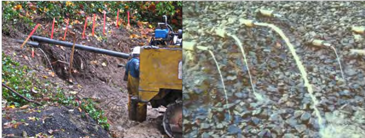
Left: Installing Horizontal drains on slopes and right: horizontal drains in operation
