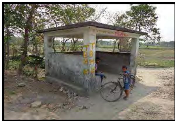
Bus shelter - Asset No C-30 in Pachim Harmati - Km 14.964 - Offset 9.3m - LHS
