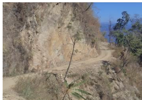
Figure 28: Landslide Prone Location along Tamenglong-Bhalok road
