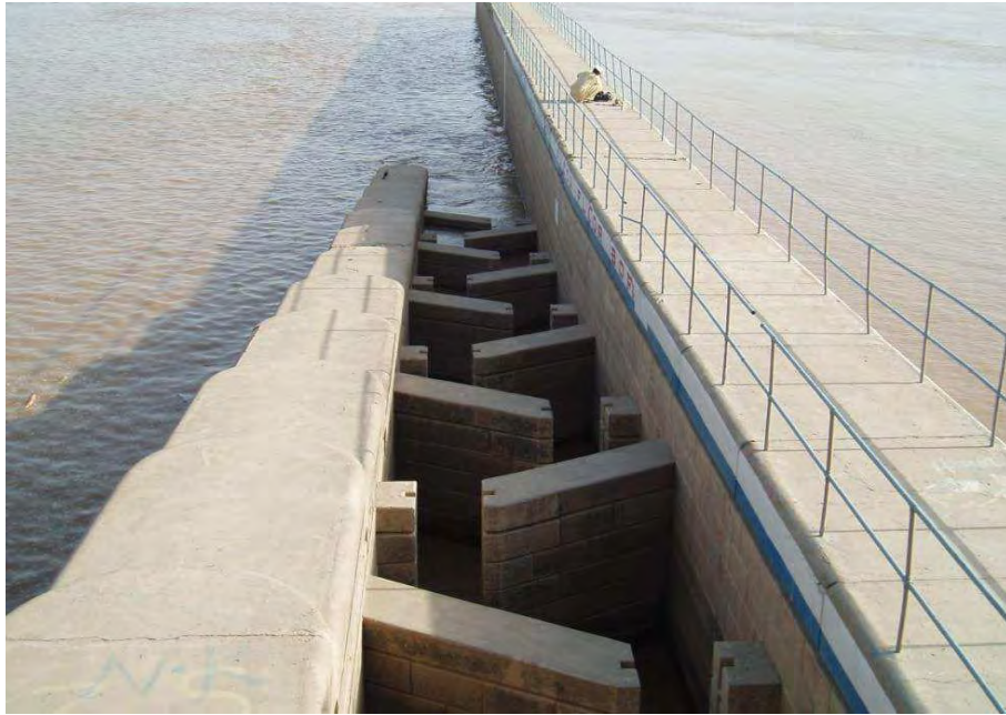
Fish Ladder along Divide Wall
