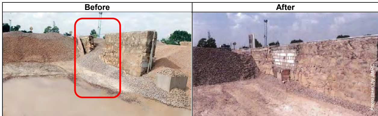
Figure 9: Broken separator wall at casting yard can lead to mixing of aggregates.
