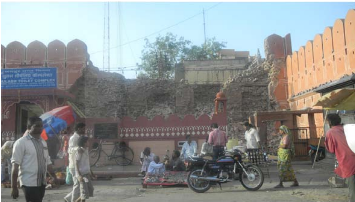
Figure 22: Monsoon Rain Damaged Section of the Wall near Chandpole Gate Showing the Use of Brick and Mud Construction Materials
