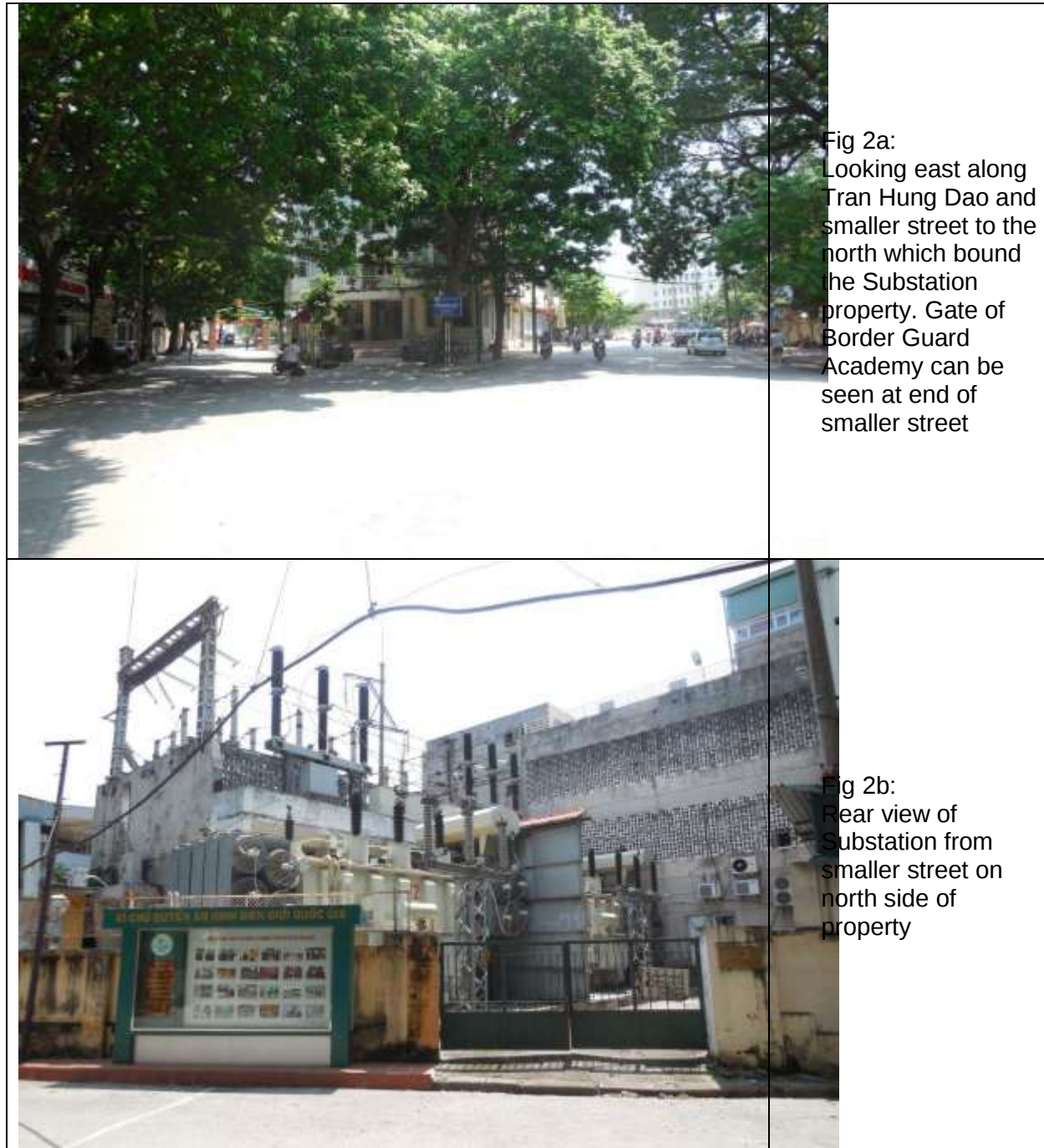
Figure 2. Views of Tran Tung Dao 110 kV Substation
